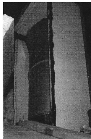
Example of an older expansion tank
