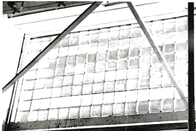
An interior shot of a completely cleaned and restored panel at 15 West Broadway.
