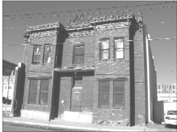
Stabilizing the Dumas was Butte CPR's biggest project ever in dollar value.
